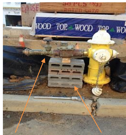
Figure 2 – Proper Hydrant Meter Support
