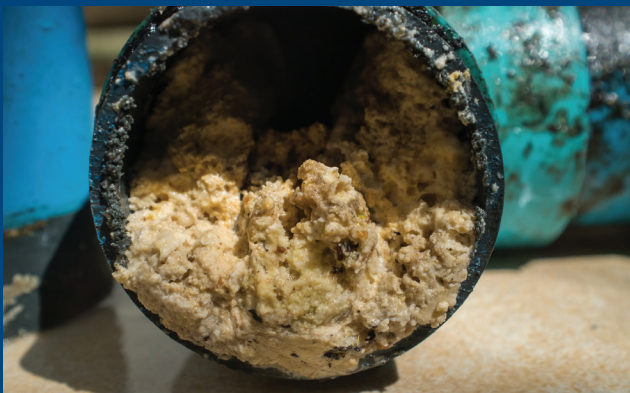
FOG Build-up in a Sewer
