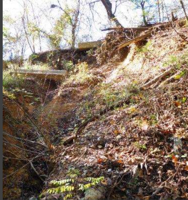
Curbs and gutters have not been maintained -- creating erosion.
