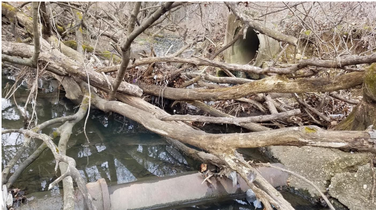
Figure 4-8: Exposed side sewer crossing 000040SEWP immediately downstream of storm water outfall
