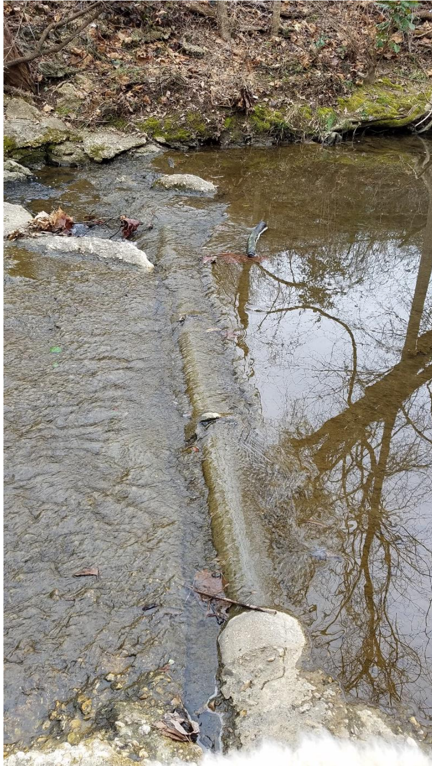
Figure 4-13: Exposed side sewer 009121SEWP on Taylor Run with damaged joints
