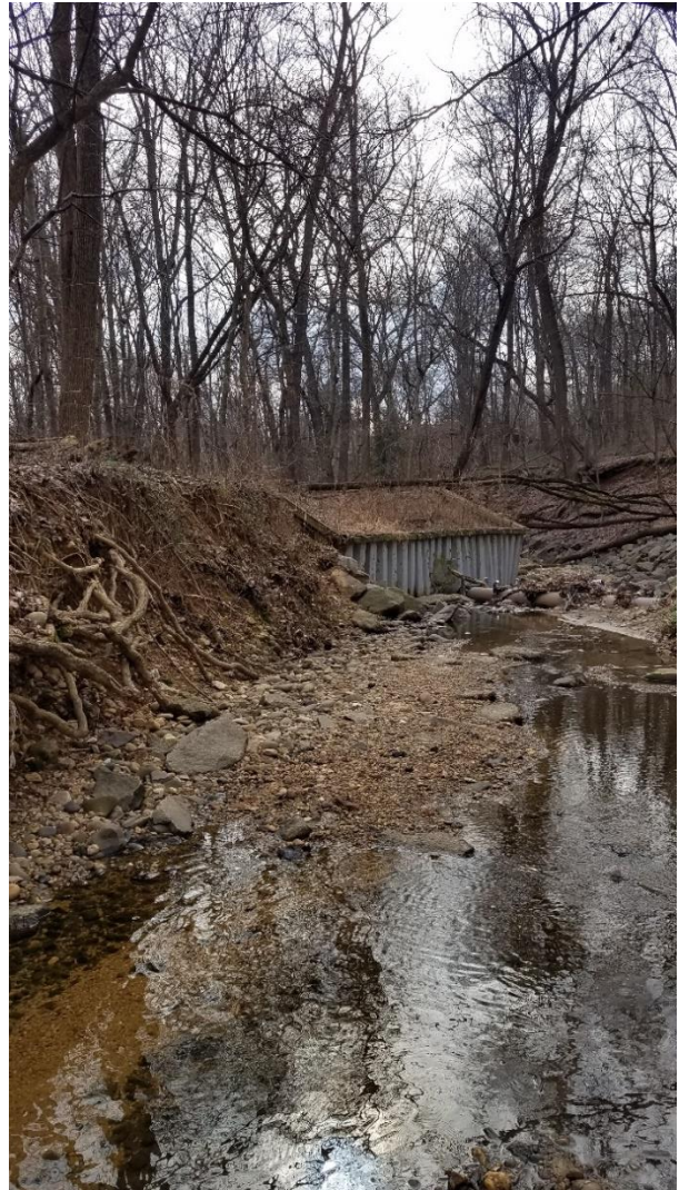
Figure 4-11: Severely Eroded Streambank upstream of crossing 009478SEWP
