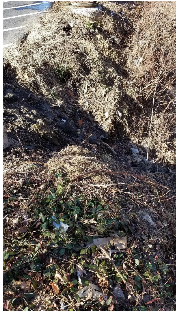
Figure 4-16: Streambank collapse looking upstream
