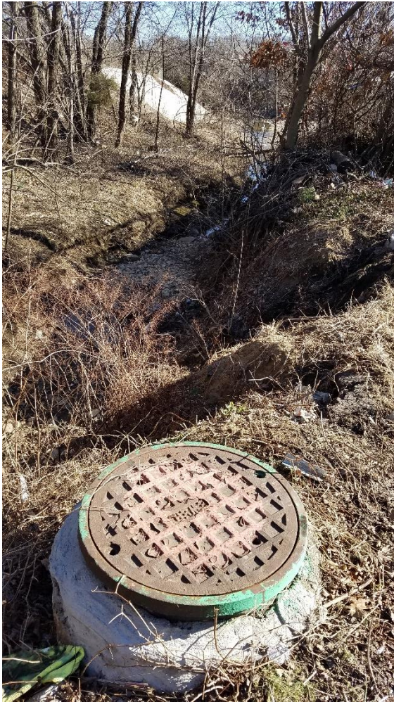
Figure 4-15: Streambank collapse at 002316SSMH
