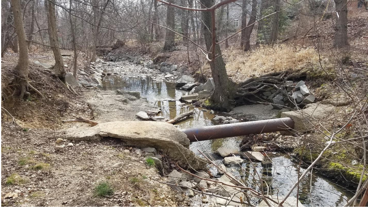
Figure 4-18: Exposed sewer 006374SEWP in Timber Branch
