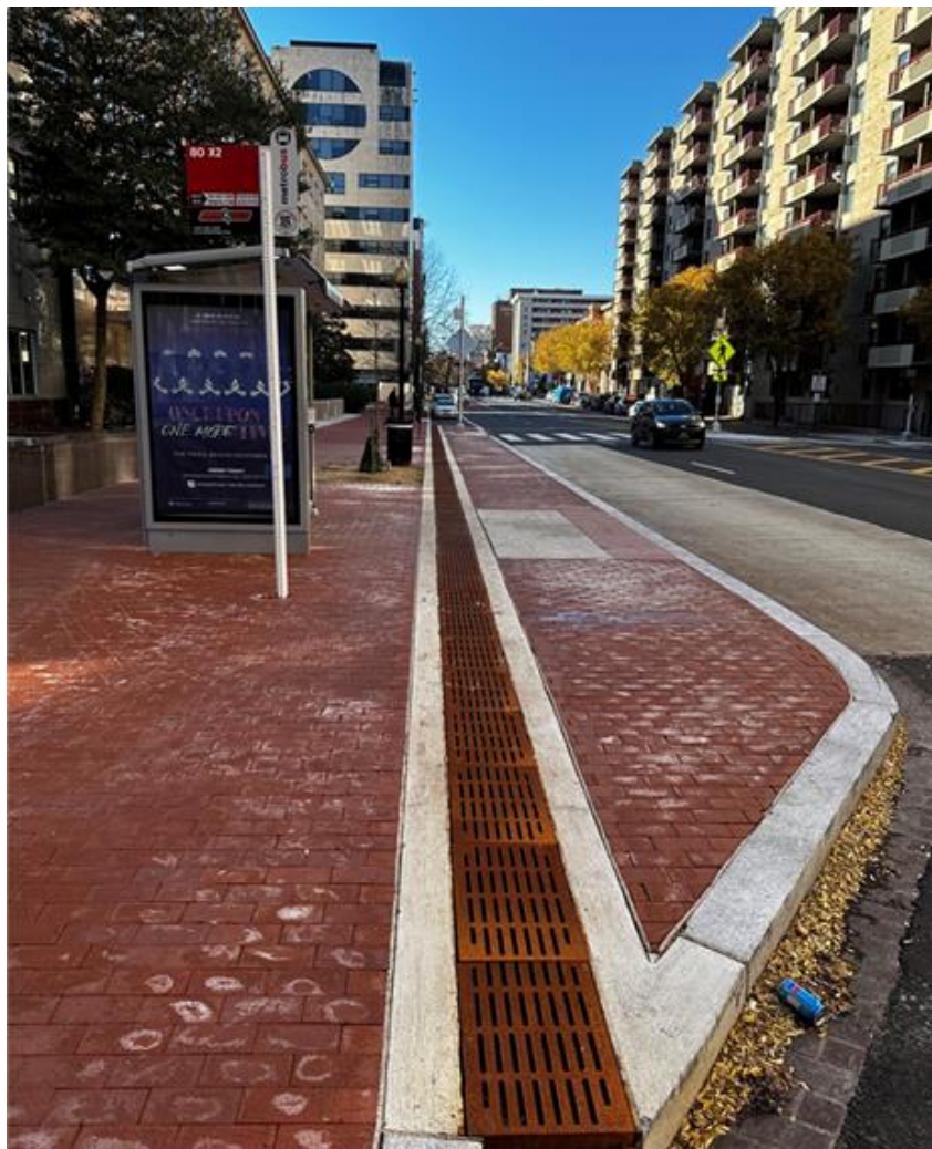
Figure 22: ADA Compliant Cover for Stormwater Trench Drain
