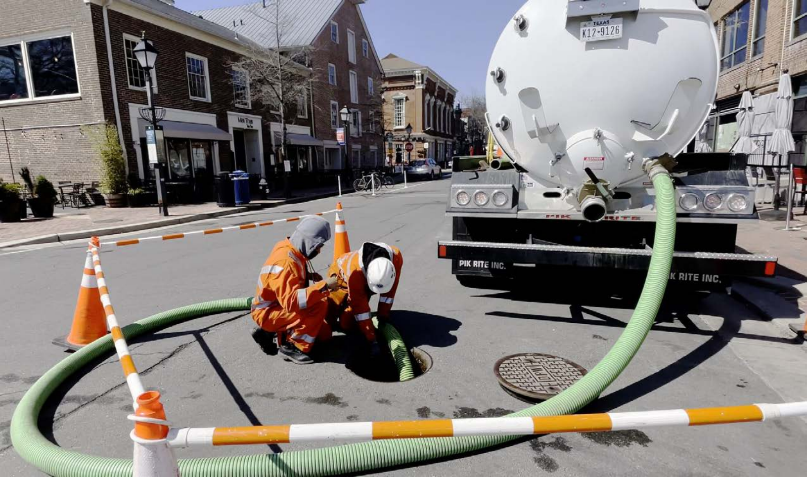
A crew uses a vacor truck to suction debris from in a storm drain as part of specialized cleaning operations on King Street on March 29. (City of Alexandria)
