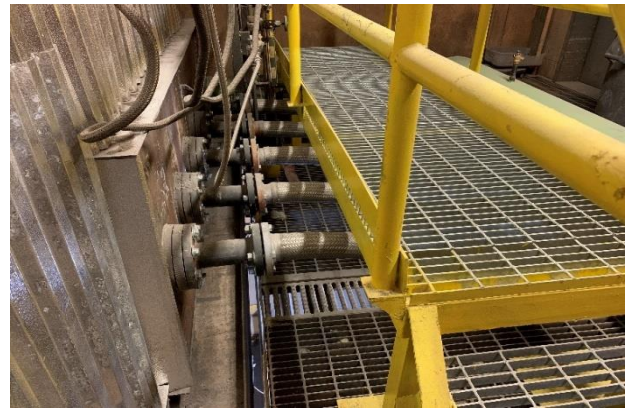
Photo: New Ammonia Nozzles on Boiler No. 1 as part of the Low NOx Technology Installation
