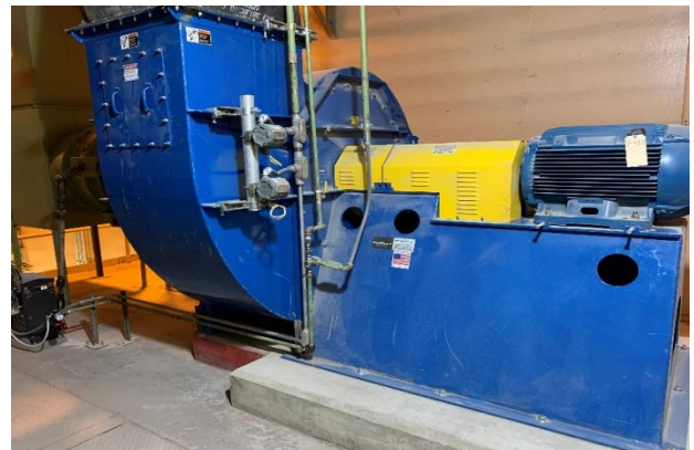
Photo: New Over Fire Air Fan on Boiler No. 1 as part of the Low NOx Technology Installation.
