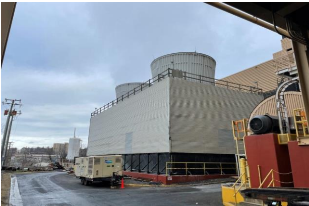
Photo: Cooling Tower
