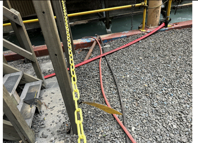
Figure 16: Temporary hoses set up to transport wastewater from the trench drains to the Cooling Tower basin
