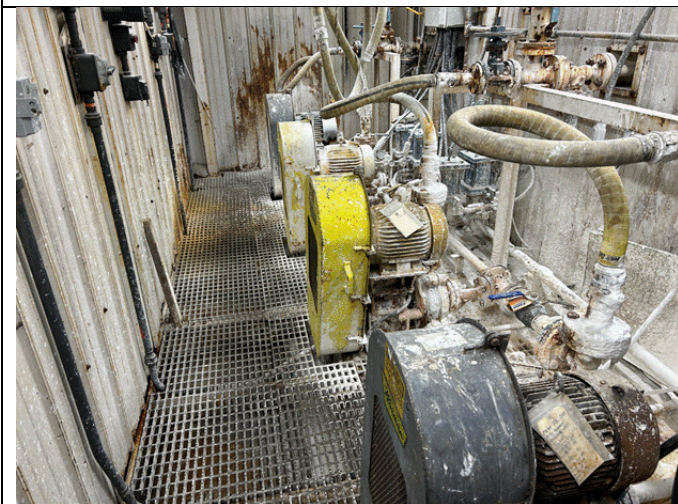
Figure 5: Lime slurry pumps
