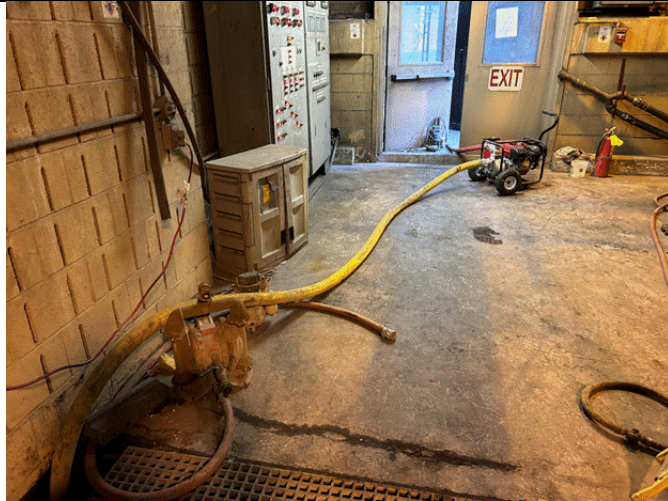
Figure 15: Temporary pump set up to transport wastewater from the trench drains to the Cooling Tower basin
