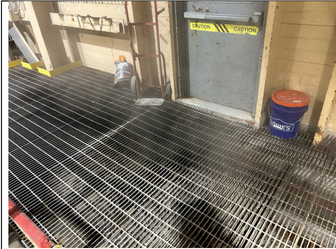
Figure 13: Leak on process pipe under platform grating.
