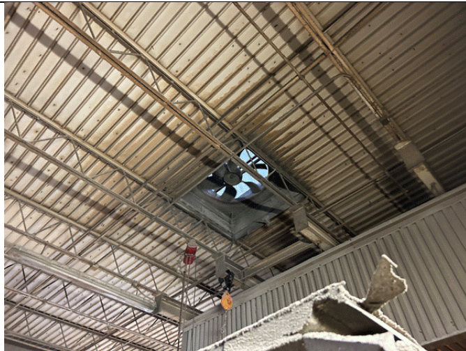
Figure 17: Boiler building exhaust fan above Boiler No. 3 not operational.
