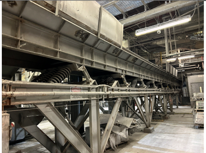
Figure 2: Ash material vibrating conveyor
