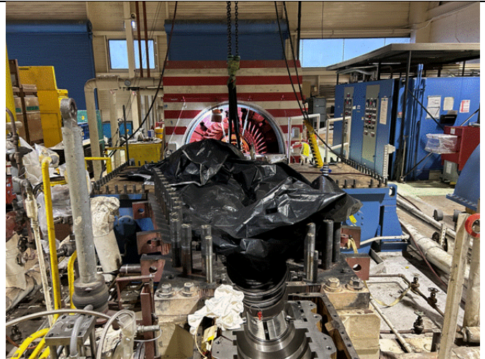
Figure 8: TG-2 disassembled for bearing damage – Turbine casing open and rotor removed
