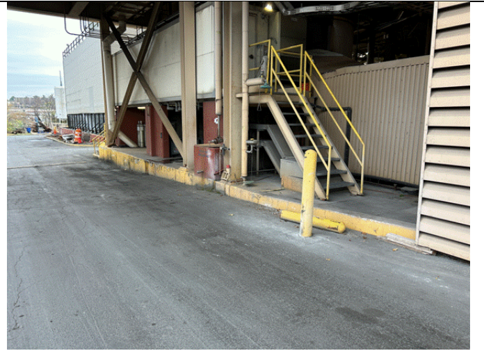
Figure 14: Bollard damaged on West side of Facility access roadway.
