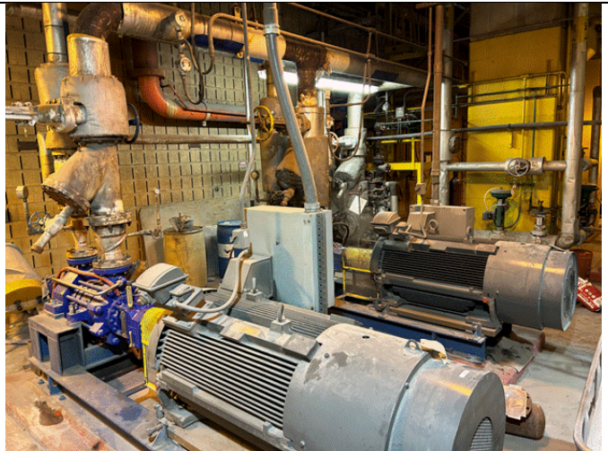
Figure 4: Boiler feedwater pumps
