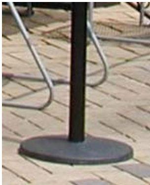
Stanchion base must be flat and no more than 1/2" above sidewalk surface
