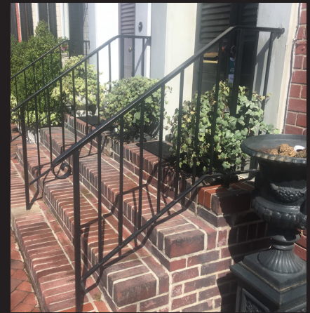
Example of inappropriate modern brick stoop and iron handrail on an Italianate style residence.
