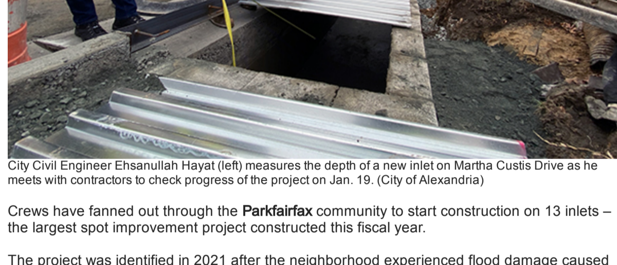
City Civil Engineer Ehsanullah Hayat (left) measures the depth of a new inlet on Martha Custis Drive as he meets with contractors to check progress of the project on Jan. 19. (City of Alexandria)
