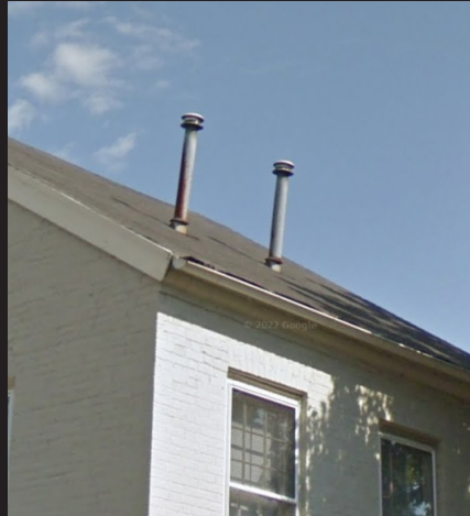
Example of an inappropriate exterior metal flue chimney on a historic building.
