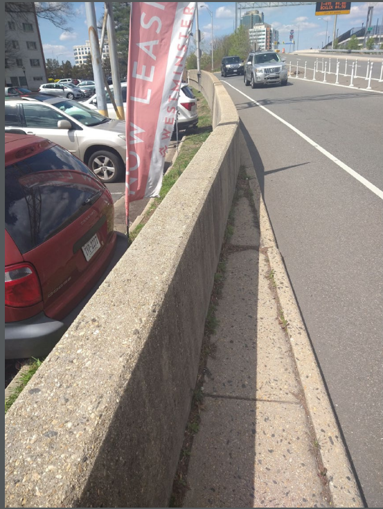
North of Kenmore Avenue, the sidewalk along the south side of Seminary Road dwindles to nothing as the road splits into multiple exit and entry ramps and bridges across I-395.
