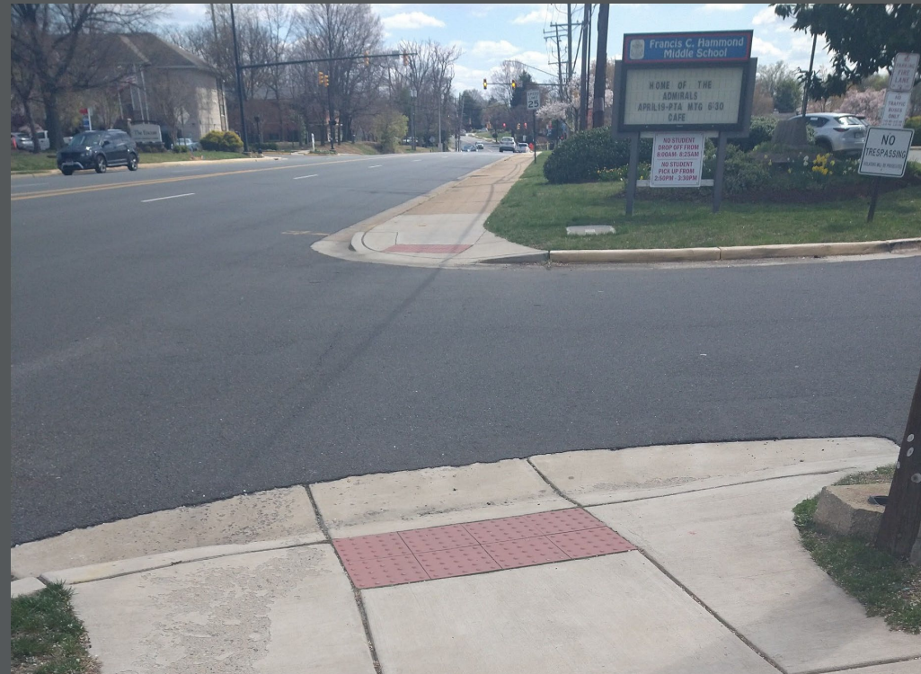
Many of the school's entranceways have detectable warning surfaces, but no crosswalk markings. Some have neither.
