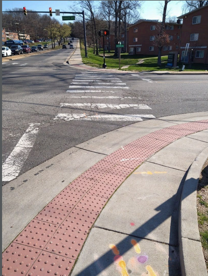
The curb radius at Beauregard Street and Sanger Avenue has been shaved back so far, the sidewalk is barely wider than the detectable warning surface. Additionally, note the cracked and faded crosswalk markings.
