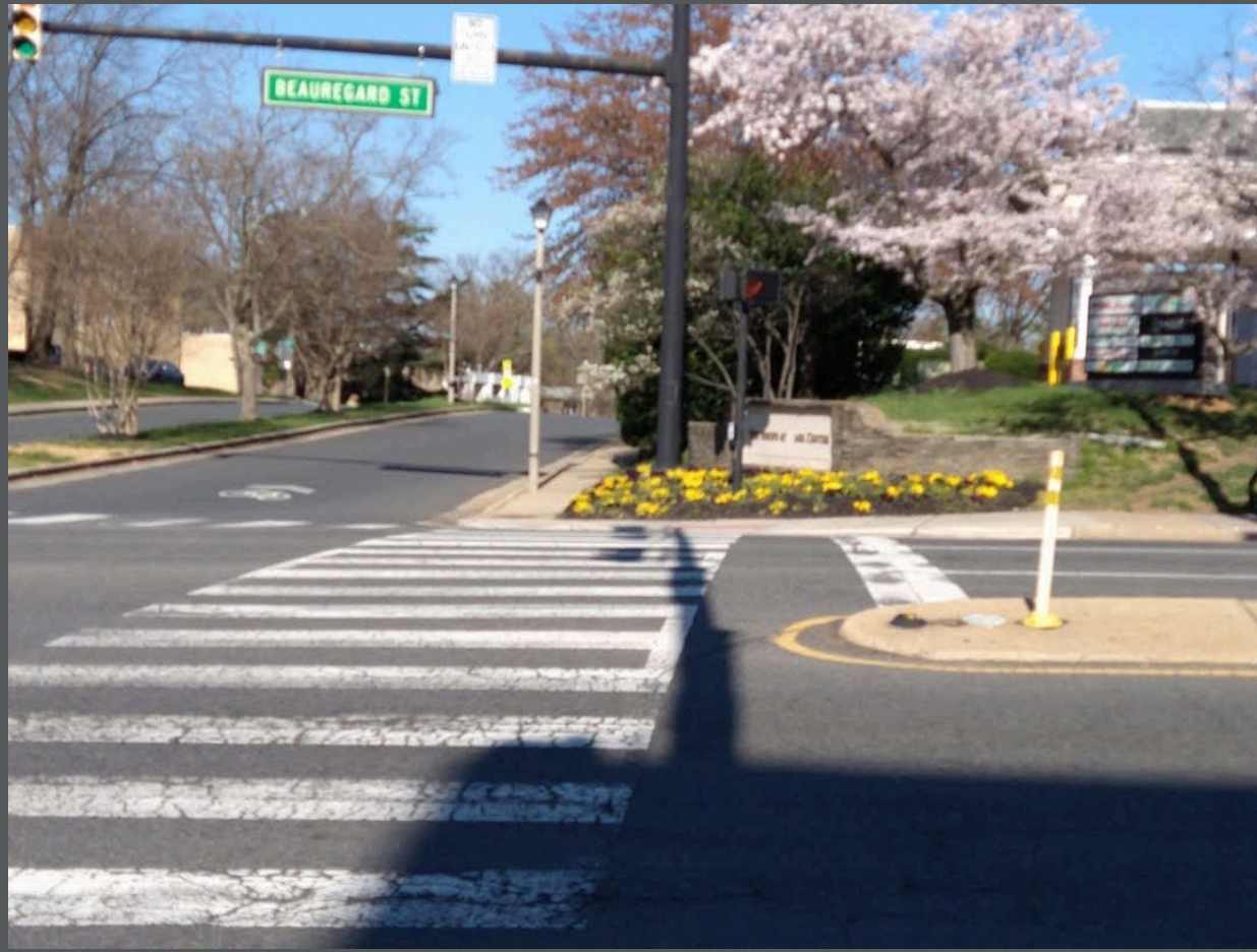
Many crosswalks along and across N Beauregard Street are cracked, faded, or some combination of the two. This is crossing Reading Avenue on the east side of Beauregard Street.
