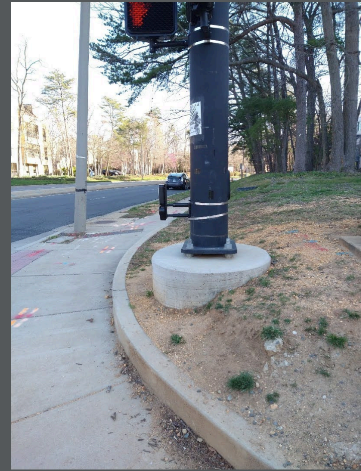
Several intersections along N Beauregard Street—this is at Rayburn Avenue—have oversized signal poles mounted on large bases away from the sidewalk, which means that, even mounted on extenders, the APS buttons are not accessible.
