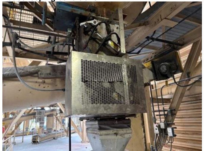
Figure 28: New Deficiency: Unit 1 SDA dump valves stuck in the open position without cage
