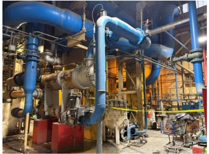
Figure 14: Maintenance observed around the condenser
