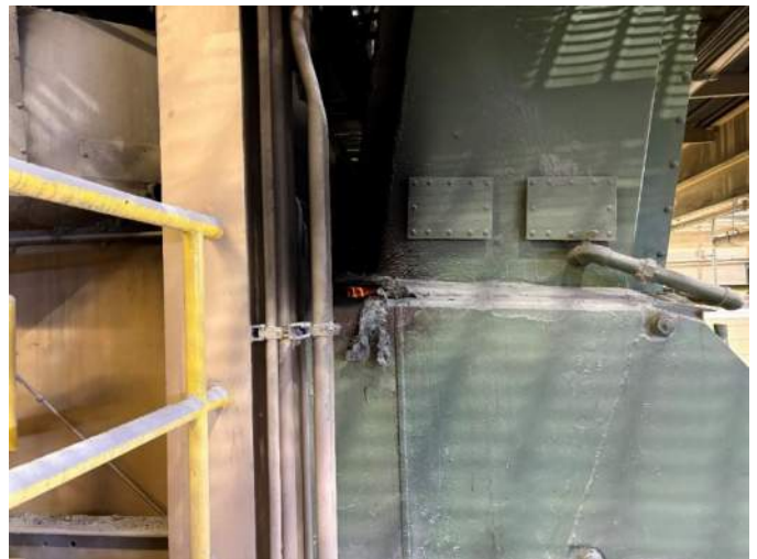
Figure 18: New Deficiency: Unit 3 hole identified in the transition chute.
