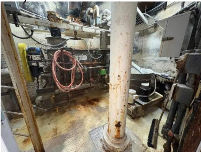
Figure 27: Lower lime silo floor corrosion
