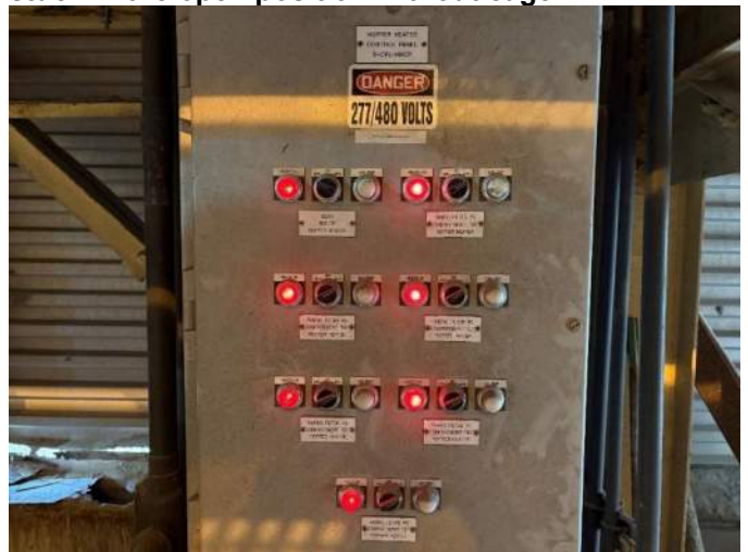
Figure 30: Updated Deficiency: Unit 3 baghouse hopper heaters; one remains in manual
