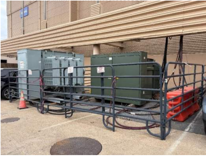
Figure 1: Temporary generator in the front parking lot
