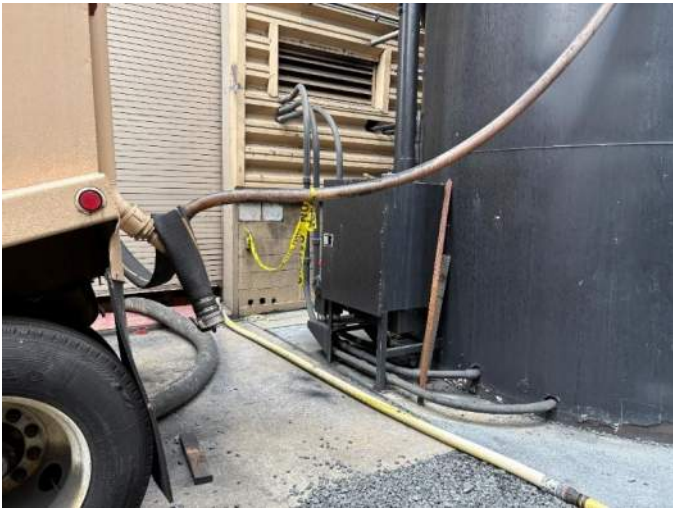
Figure 5: Maintenance observed around Carbon Silo hoses
