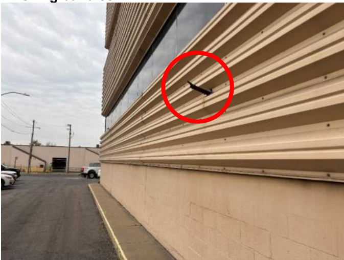
Figure 11: New Deficiency: External deodorizer not working
