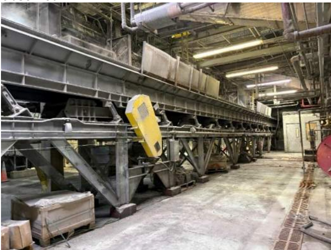
Figure 15: Vibrating conveyor area housekeeping in good condition
