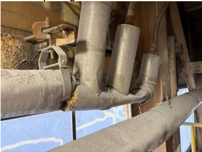
Figure 23: Updated Deficiency: Damaged insulation has worsened; new leak observed on the North side of Unit 3
