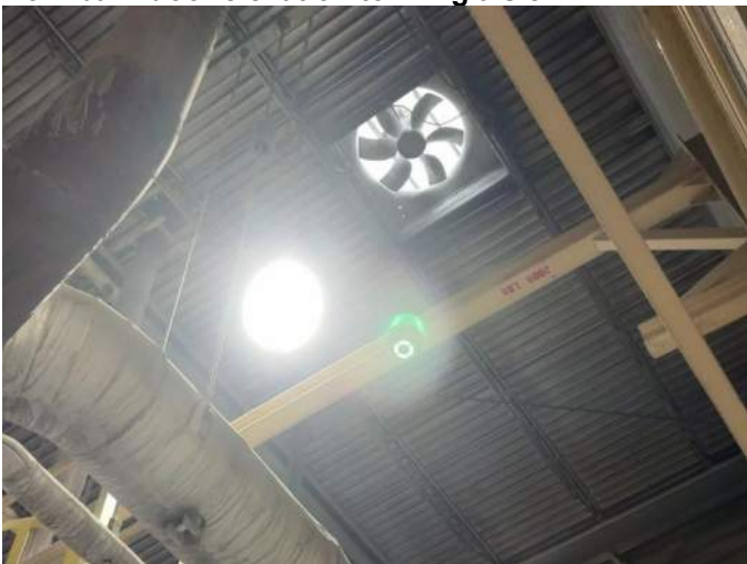
Figure 21: Updated Deficiency: Fan above deaerator observed operating
