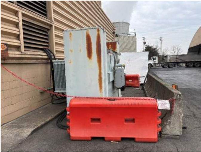
Figure 7: Temporary generator on North side of Facility
