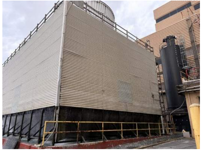
Figure 2: Cooling tower appears to be in good condition
