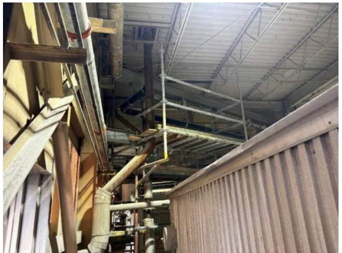
Figure 22: New silencer installed on steam vent piping
