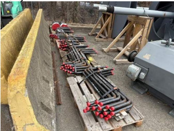
Figure 9: Unit 3 superheater tie ins for the primary and finishing bundles
