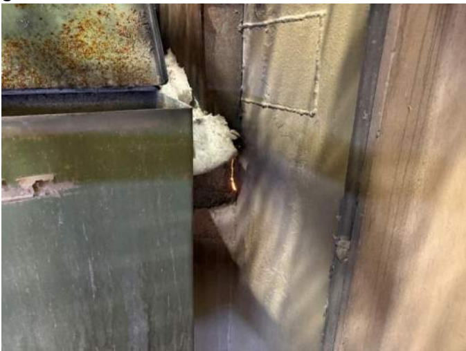
Figure 17: New Deficiency: Unit 2 transition chute shows previous repair and new crack in wall
