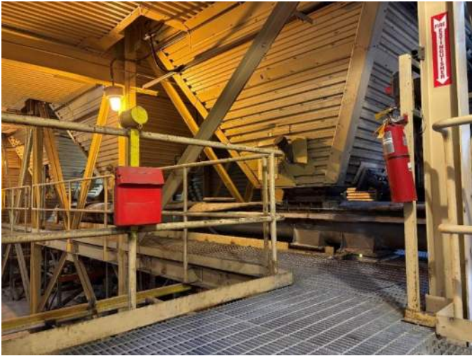
Figure 25: Unit 2 baghouse hoppers and screw conveyors – no issues observed
