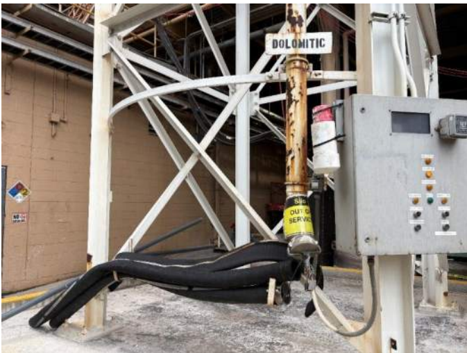
Figure 3: Dolomitic lime silo fill pipe marked out of service
