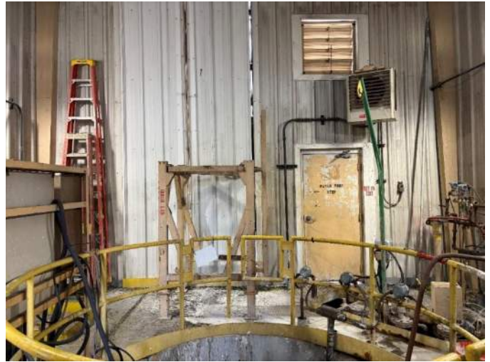
Figure 26: Unit 3 SDA Penthouse Enclosure - poor housekeeping conditions
