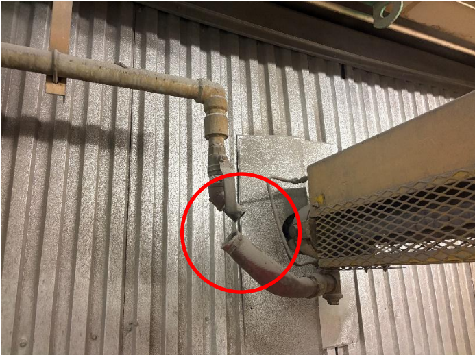
Figure 17: Boiler No.2 IK-08 Sootblower Disconnected – New Deficiency
