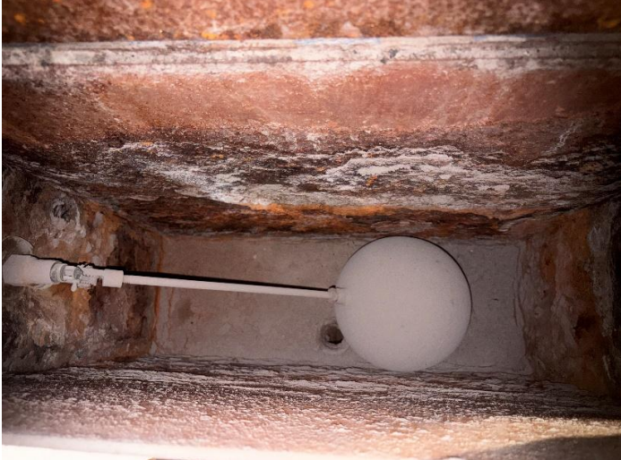
Figure 15: Boiler No. 1 Water Box Empty – New Deficiency
