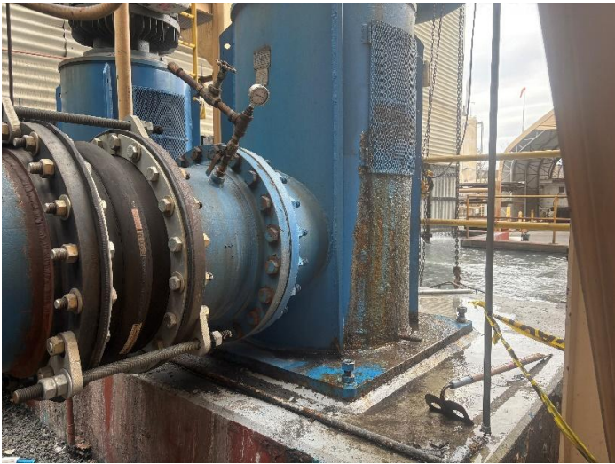
Figure 3: Circulating Water Pump on East Side of Cooling Tower
