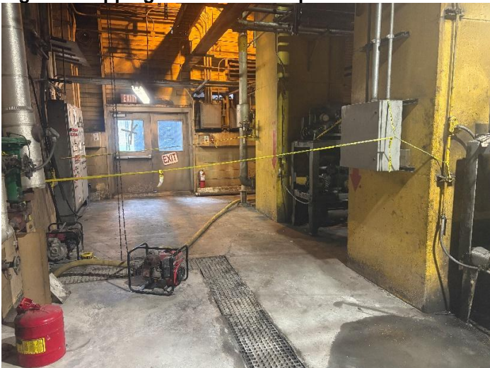
Figure 11: Temporary Pump set up to transport wastewater from the trench drains to the Cooling Tower basin. Punchlist item since 2022.
