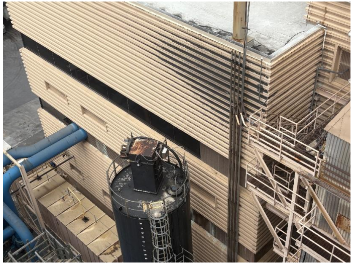
Figure 22: Carbon on External Side Wall – New Deficiency
