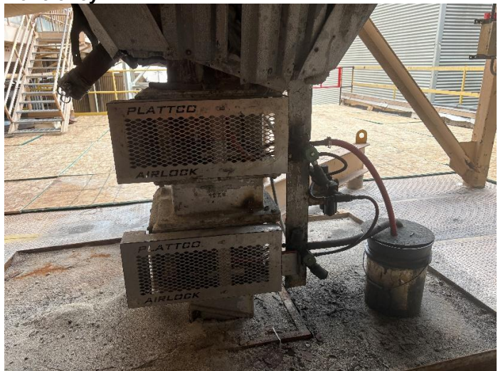
Figure 24: Unit No. 1 Economizer Plattco Covers
