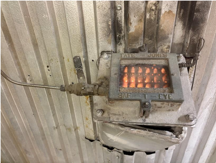
Figure 19: Air Shut Off to Several Viewports on Boilers – New Deficiency
