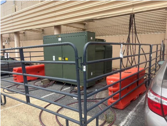
Figure 1: Temporary Generator in Front Parking Lot
