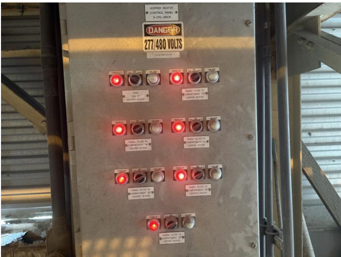
Figure 23: All Baghouse No. 3 Heaters on with no Low Temp Indicators. (No change to Deficiency #8)
