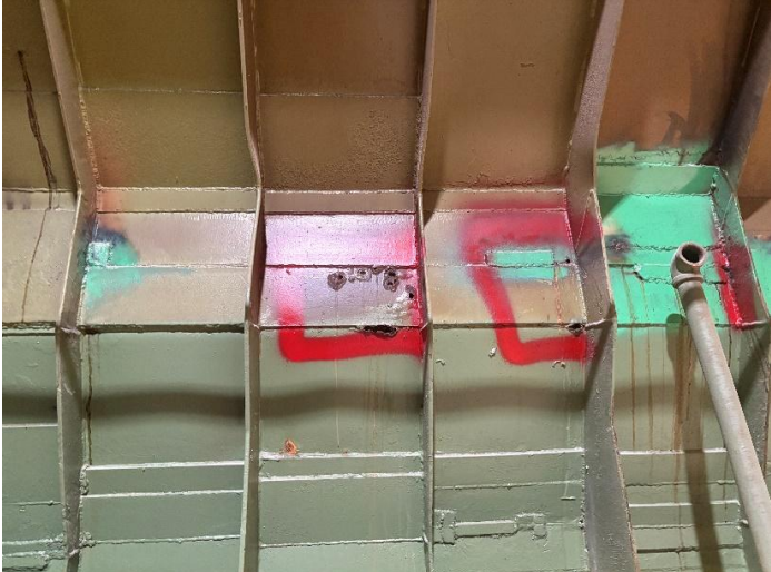
Figure 16: Boiler No. 3 Feed Chute marked for repairs
