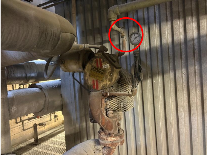
Figure 18: Boiler No.2 G9-B11 Sootblower Disconnected – New Deficiency
