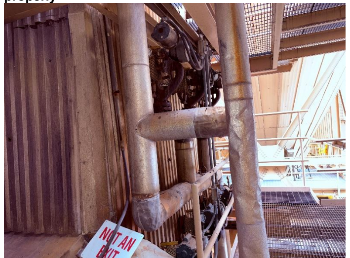
Figure 12: General observation of economizer sootblowers
