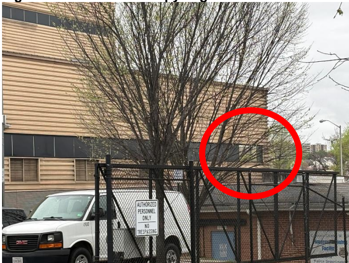
Figure 5: Missing window in tipping hall
