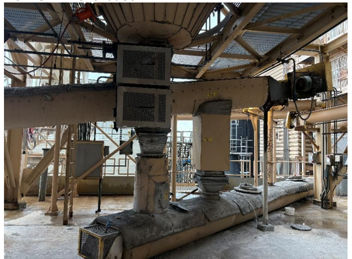
Figure 24: Baghouse screw conveyors on Unit No. 3
