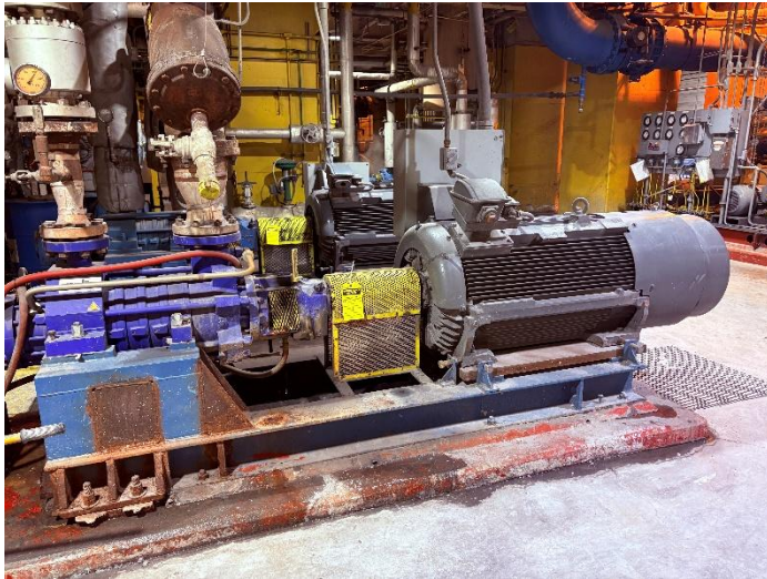
Figure 7: General photo of boiler feedwater pumps
