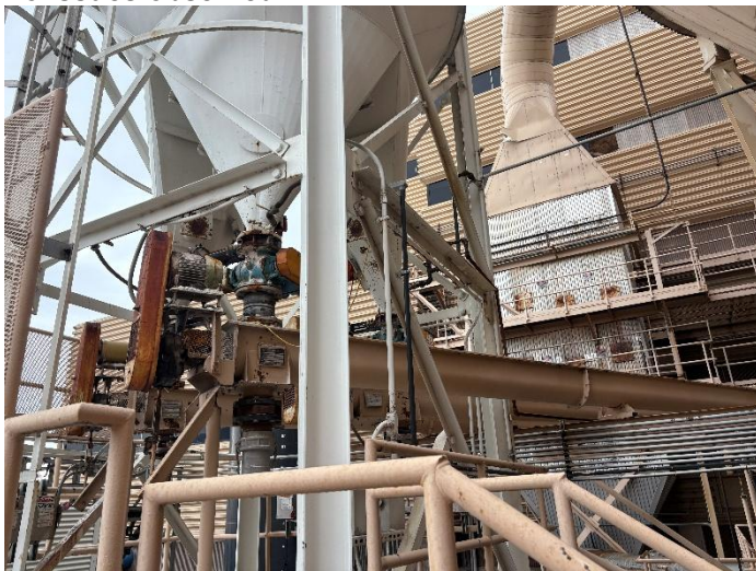
Figure 23: Lime silo hopper and screw conveyor – No issues observed
