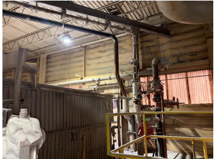
Figure 20: New silencers installed on Boiler No. 3
