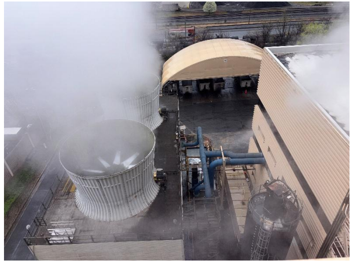
Figure 22: Cooling Towers, and ash trailer canopy from SDA Penthouse
