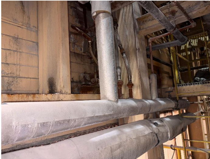
Figure 19: Deficiency Item 0625-2 leak and hanger repaired
