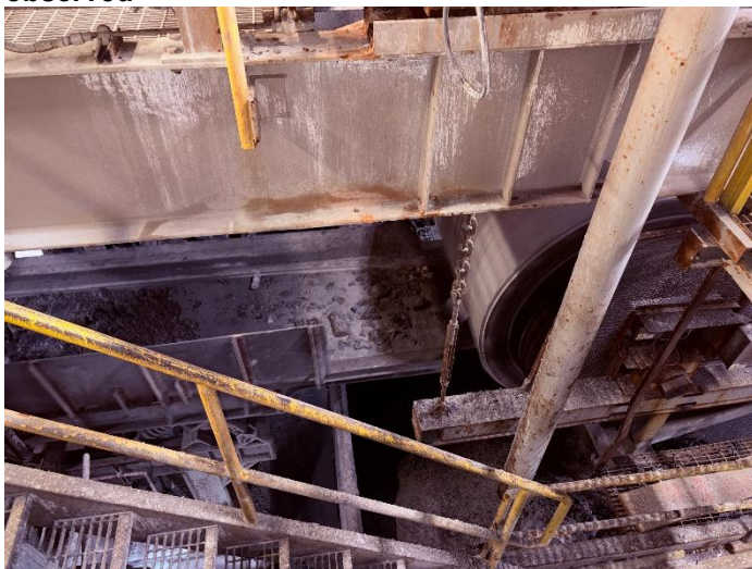
Figure 11: Ferrous collection system – no issues observed
