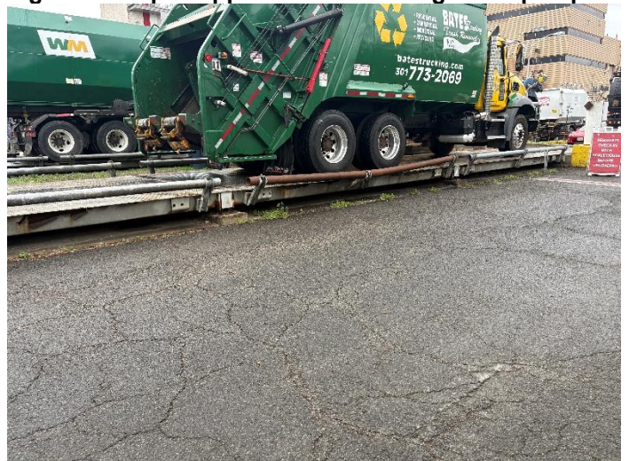
Figure 4: Side bar of scale is damaged
