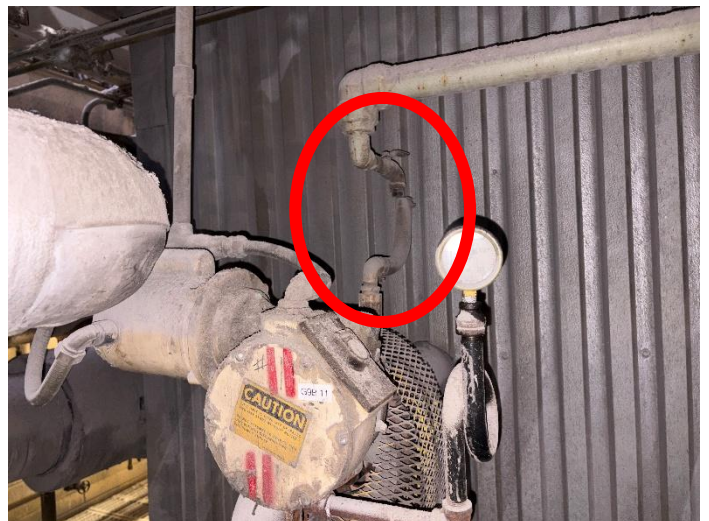
Figure 18: Unit 2 G9B-11 sootblower seal air disconnected
