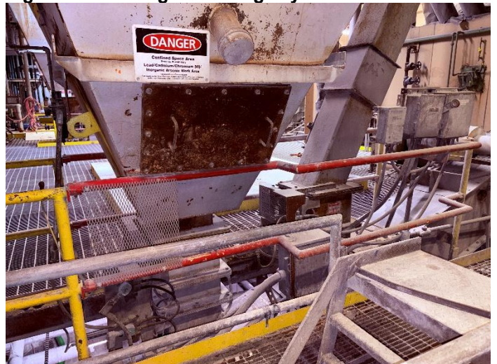
Figure 10: All superheater dump valves working properly
