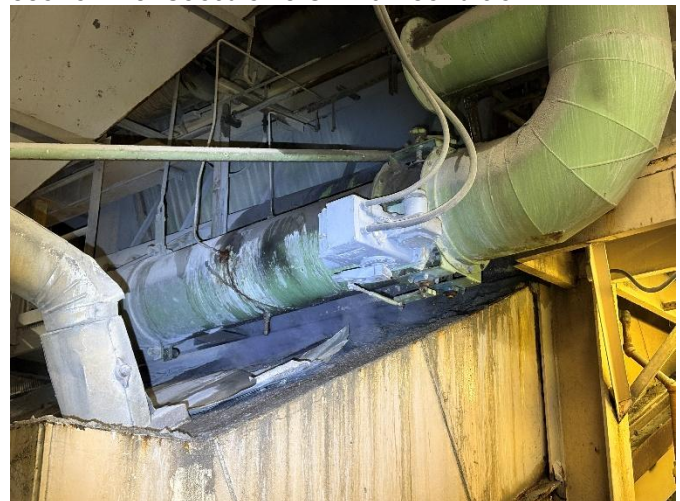
Figure 10: Steam leak on Boiler No. 3 – Repaired the following day
