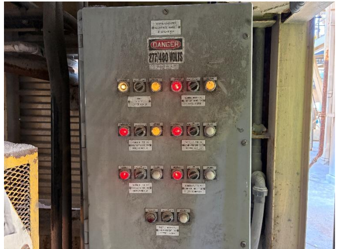
Figure 18: All hopper heaters observed in the "auto" position
