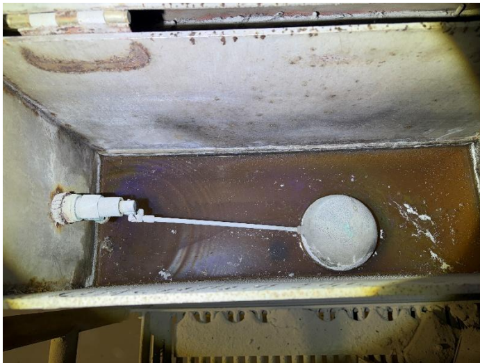
Figure 7: Water level boxes across all Boilers were observed full.
