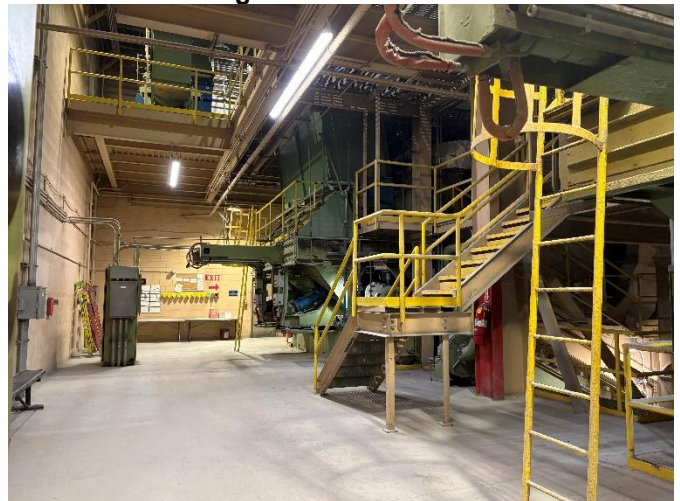
Figure 6: Firing Aisle - No issues observed
