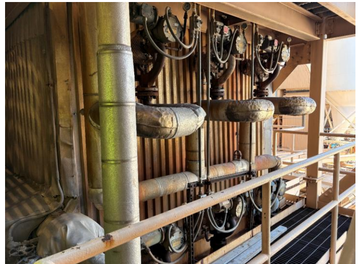
Figure 8: General observation of Boiler No. 3 economizer sootblowers in fair condition.
