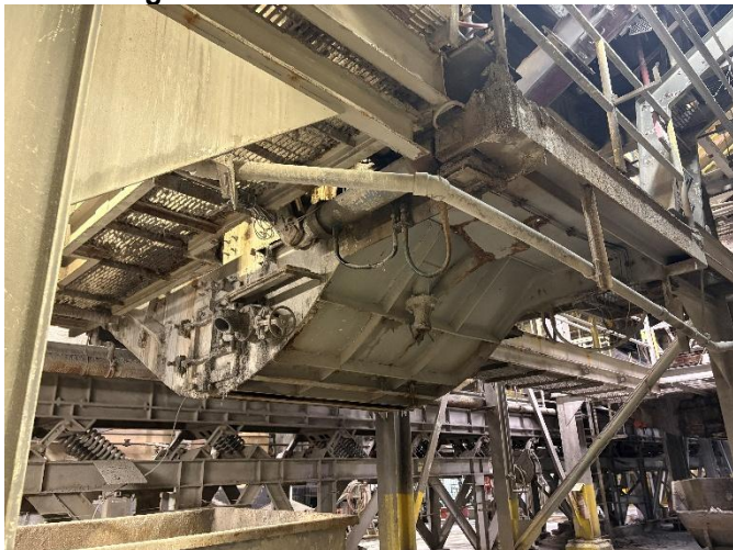
Figure 5: General observation of Boiler No. 3 ash discharger in good condition
