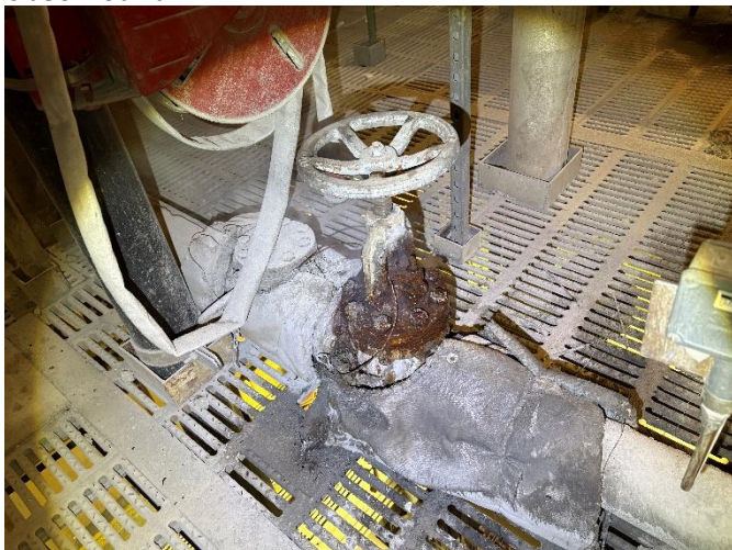
Figure 9: Deficiency Item 0626-02 – Boiler No. 2 attemperor isolation valve leak
