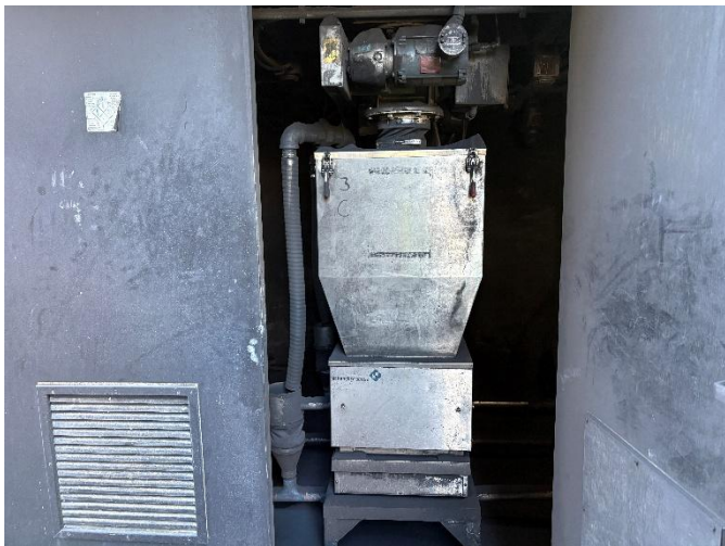
Figure 3: General observation of carbon silo feeder, clear of fugitive dust.
