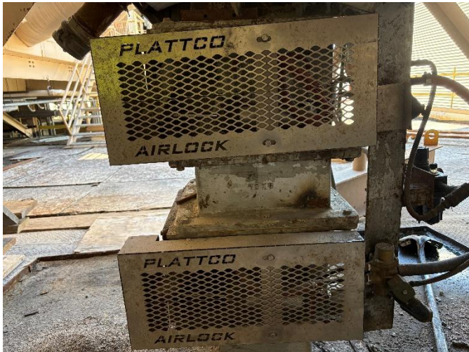
Figure 17: Deficiency Item 0126-01: cages around Unit 1 SDA Double-Dump Valves repaired
