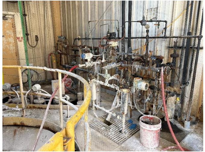
Figure 14: General housekeeping conditions in Unit 3 SDA penthouse
