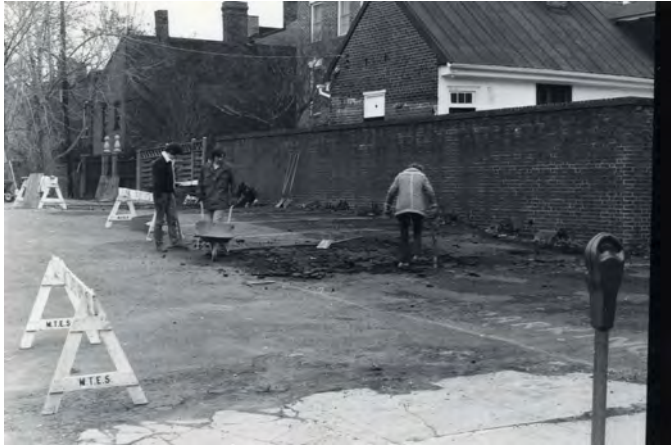
Fig. 4: Phase I of the excavation, excavating the parking lot (ALEXANDRIA ARCHAEOLOGY COLLECTION)
