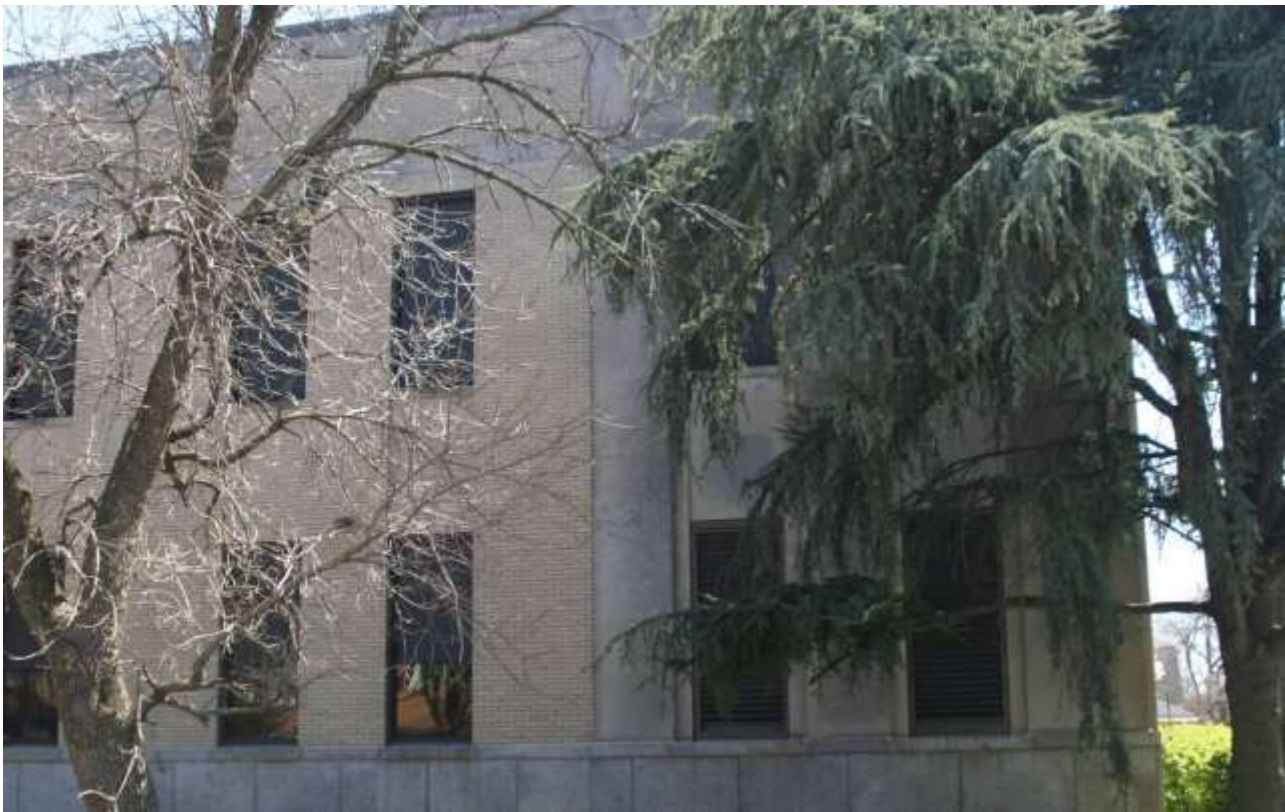
4. 1316 Mt. Vernon Avenue. North elevation, detail last bay, straight angle, facing S. Photograph by Gwen White, 4/6/14.
