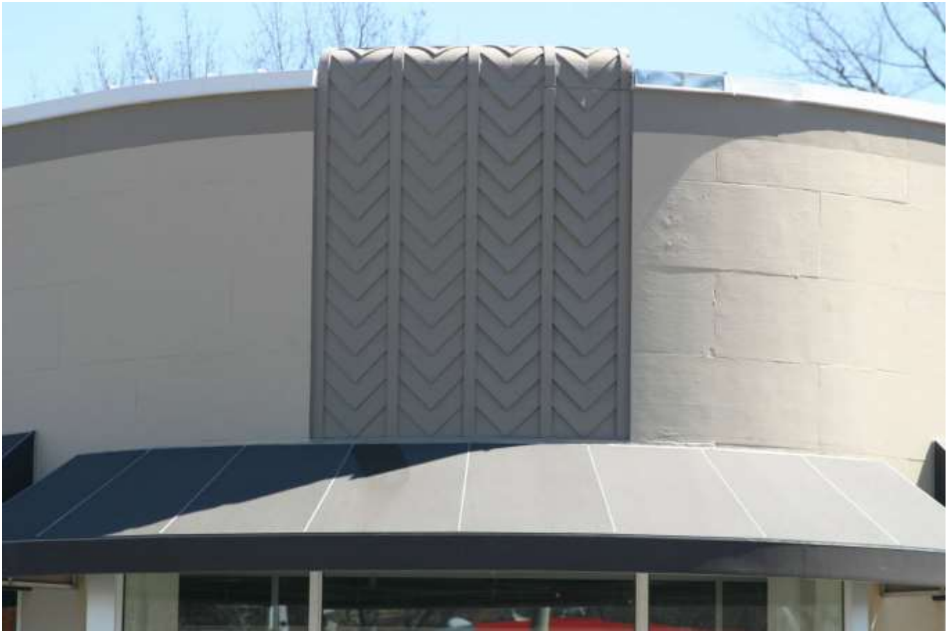
3. 1509-1517 Mt. Vernon Avenue. Façade, detail chevron keystone above entrance, oblique angle, facing 125° SE. Photograph by Gwen White, 4/6/14.
