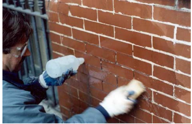
Fig 10. Once all mortar has been removed from the joints, wash away dust and particles with water and a brush. This helps in two ways: It prevents replacement mortar adhering to masonry, it also prevents shrinkage crack formation (the brick will not absorb water from the mortar). Before installing material, eliminate standing water.
