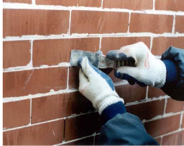
Fig 2. To ensure that the brick is not damaged when the mortar is removed, it is necessary to find the joint. In the most sensitive manner possible, gently scrape off the mortar adhered to the face of the brick.
