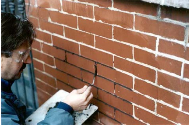
Fig 13. With the bed (horizontal) filled, the size of the vertical openings will be reduced and less material is needed to be inserted into them (upper left). If joints are very deep, fill them to a uniform level below the surface and allow it to set. When you return to complete the pointing, abrade the already installed mortar to remove the thin, waterproof skin that has formed on the exterior. Install a second layer of mortar. In all cases, fill the joints with slightly more mortar than necessary.
