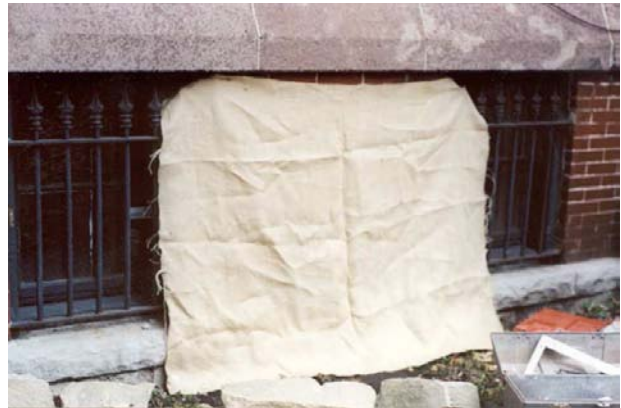
Fig 16. Following mortar installation protect the area from the sun, wind, and rain, with burlap and/or plastic sheeting to allow the mortar to cure slowly through carbonation. To impede drying, joints need to be moistened periodically during the first 72 hours. The rate of mortar drying depends on environmental factors: temperature, level of humidity, and direct sunlight exposure. You may need to wet hot and dry
