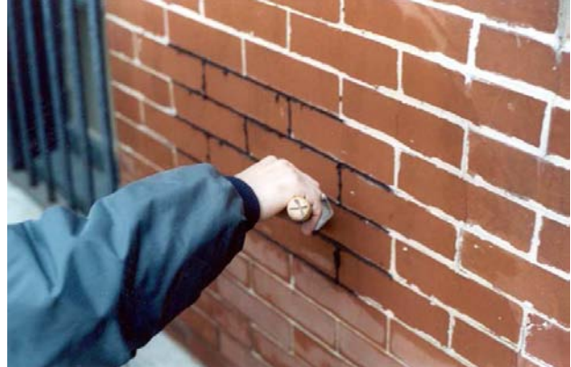
Fig 14. Once the mortar has reached thumb-print firmness, tool in the same fashion as the original, cutting off the excess with a trowel. A stiff bristled churn brush should be used to further compact the newly installed mortar and expose the aggregate.
