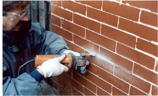
Fig 8. The mortar pictured being removed was particularly hard and the joints were very thin. After attempting to use several different tools, a caulking cutter and a diamond blade proved to work best. When cutting, be careful not to cut too deeply, through all of the mortar. Butter joints were originally laid with mortar only on the edges of the brick.
