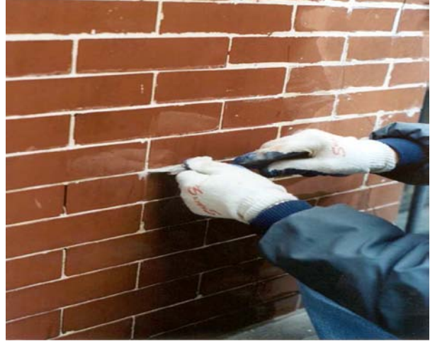
Fig 6. For mortar removal, choose the technique that makes the least impact on the masonry. The use of hand tools is always recommended. Grout keys work well to remove mortar from butter joints unless they are extremely thin.
