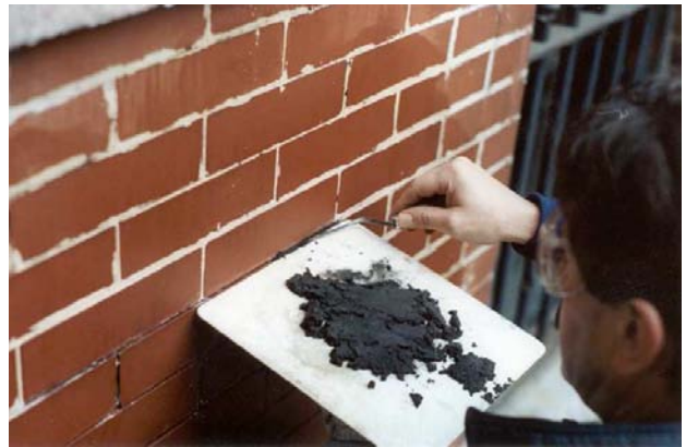
Fig 12. Using a trowel, press the mix into the hawk repeatedly to make the mix more plastic and workable. Right-handers move right to left. Slide the mortar off of the hawk into the mortar joint. To assist compaction, press the mortar in the joint at approximately a 35° angle, depositing the mortar on the brick or newly installed material to the side. Fill all bed (horizontal) joints before filling head (vertical) joints.
