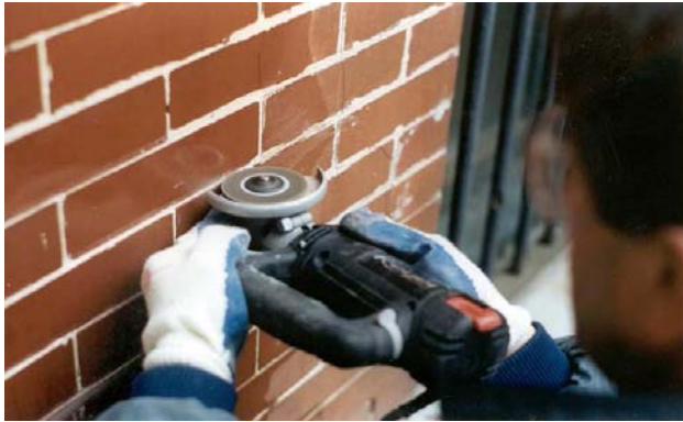
Fig 7. If the repair mortar is too hard and rigid to be removed manually, experiment with power tools. If a grinder must be used, use it only to score the center of the joint to weaken the material (above). Mark the center of the joint with a pencil and straight edge to give you a line to follow. Be certain that the diamond blade is no more than 1/2 the width of the mortar joint. Do not cut the head (vertical) joints with the grinder, only the bed (horizontal) joints. Position your hand or forearm against the wall to control the movement of the grinder.
