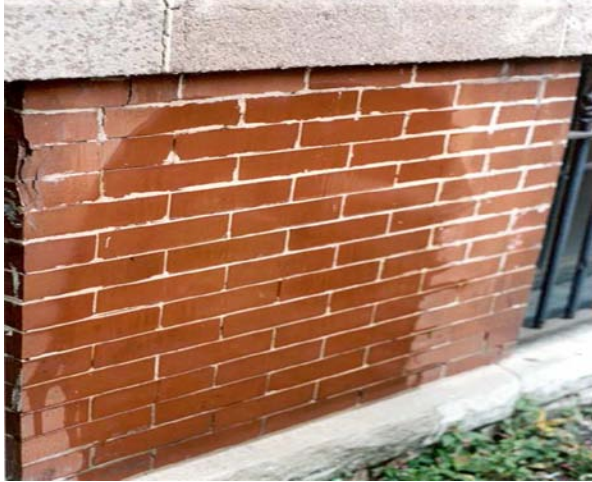
Fig 5. Thoroughly saturate the wall with water; by doing so, the lime present in the original mortar is softened, making the mortar easier to remove.
