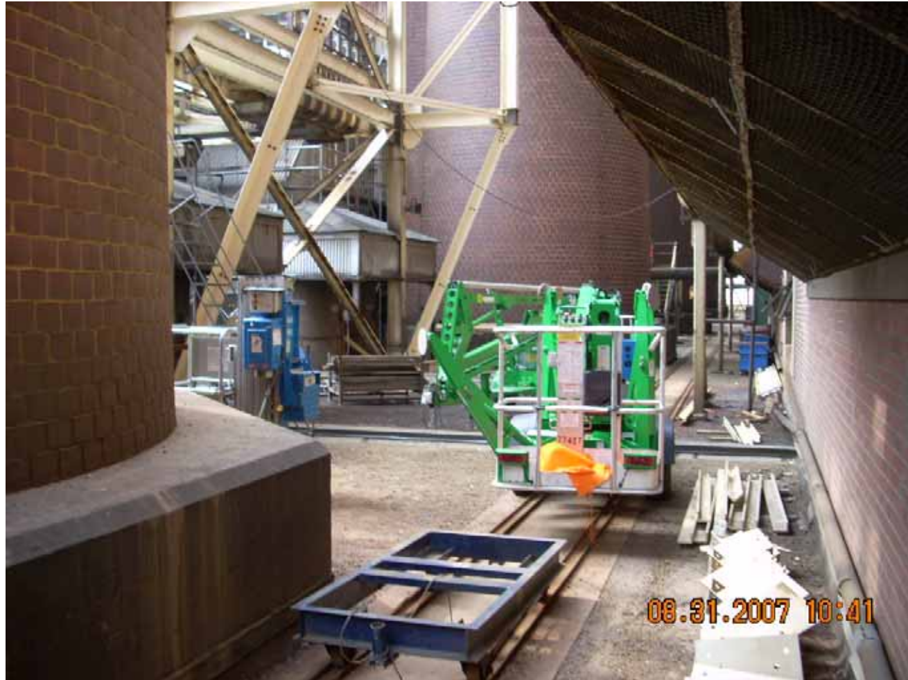
Equipment staged at the base of Stack #4 and #5.
