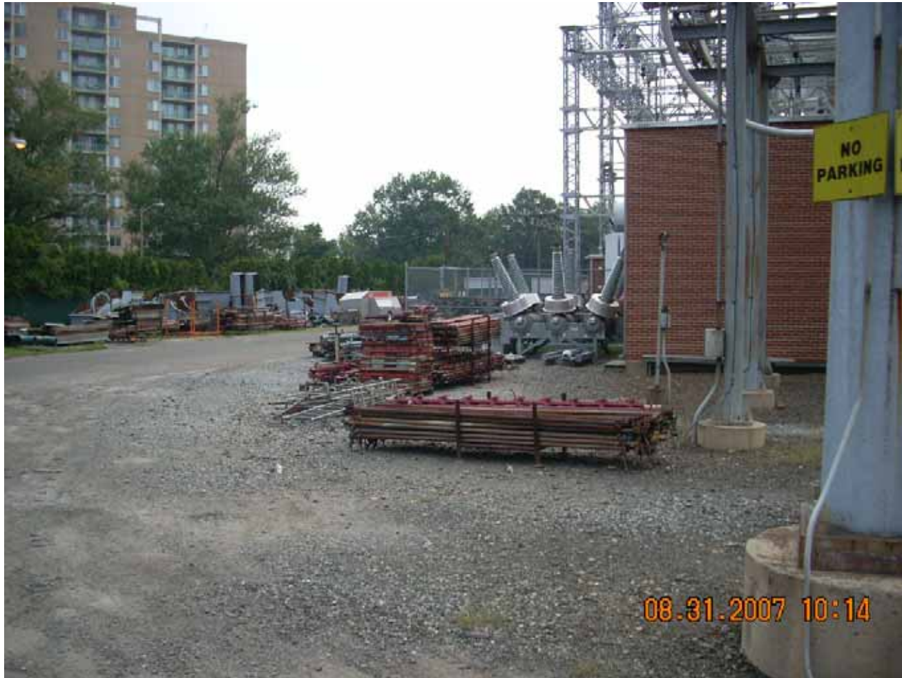
View of scaffolding and equipment staged on the northern fence line of the facility.
