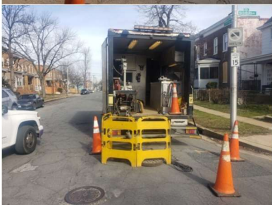
Example of typical CCTV inspection truck setup. In order to conduct CCTV inspections two trucks are needed, one at either end of the sewer.
