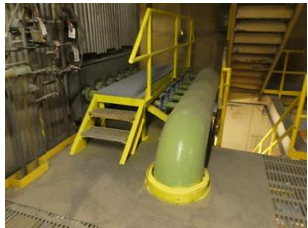
Photo: New Nozzle Installation in Upper Elevation of Boiler No. 2 as part of the Low NOx Technology Installation.
