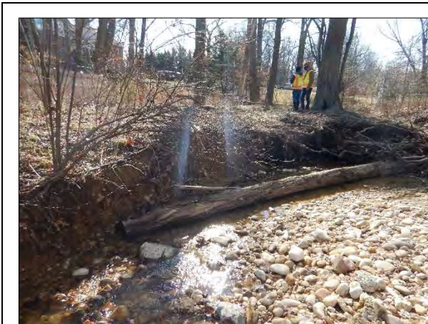
Figure 78. Downed Tree (January 2021, Station 2+20)
