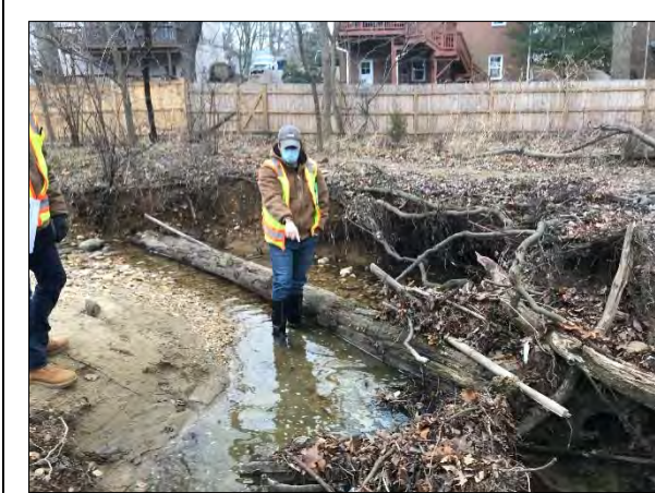
Figure 76. Downed Tree (January 2021, Station 1+90)
