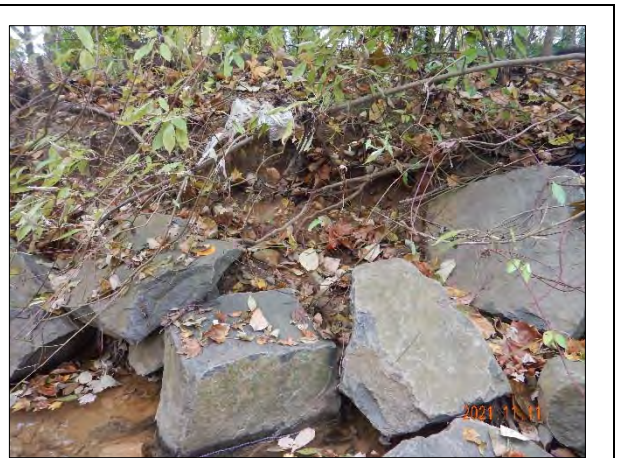
Figure 6. Displaced Rock Toe Material (Station 1+60)
