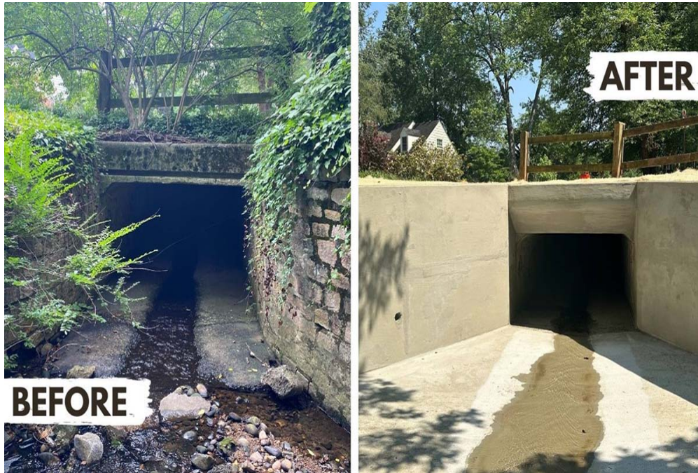
Before and after: Photos of completed culvert repairs at Timber Branch headwall.
